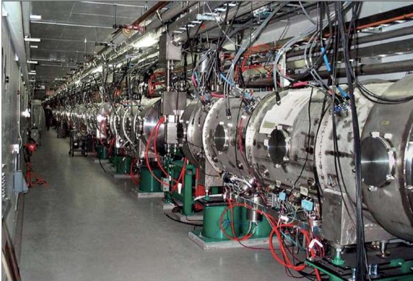
The superconducting RF proton linac at the SNS at Oak Ridge National Laboratory is providing valuable experience for a future ADS accelerator. Image credit: ORNL.
